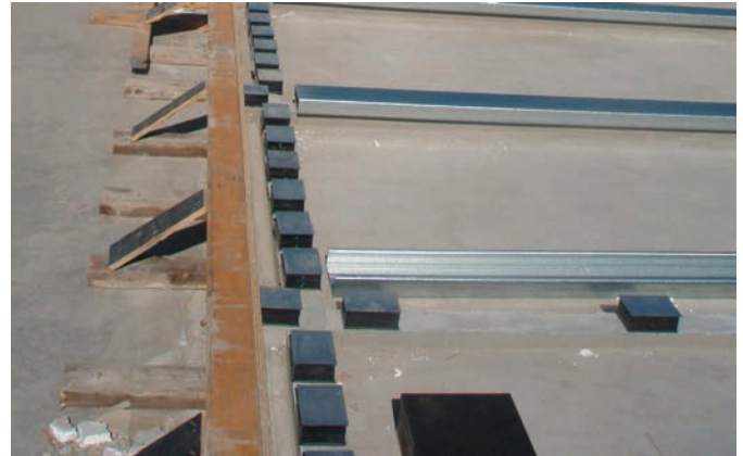
ISOLATION BEARINGS, CHANNEL 7 STUDIOS SYDNEY
